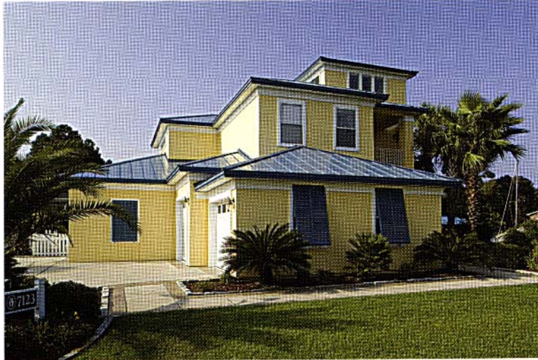
An infrared-reflective coating was applied to this stucco home in Panama City, FL. Photo courtesy of Textured Coatings of America
